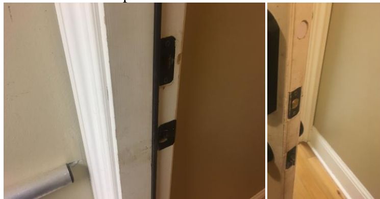
Close Up of Latch Receiver in Door Jam and Latch on Edge of Door
