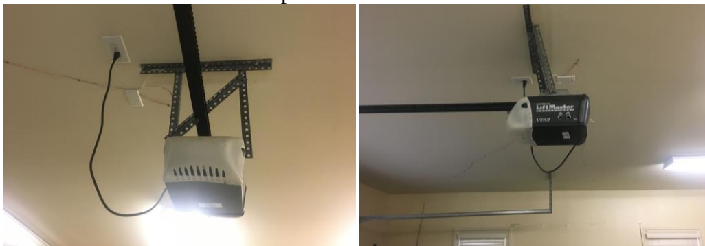
Motor – showing Plug in Ceiling
